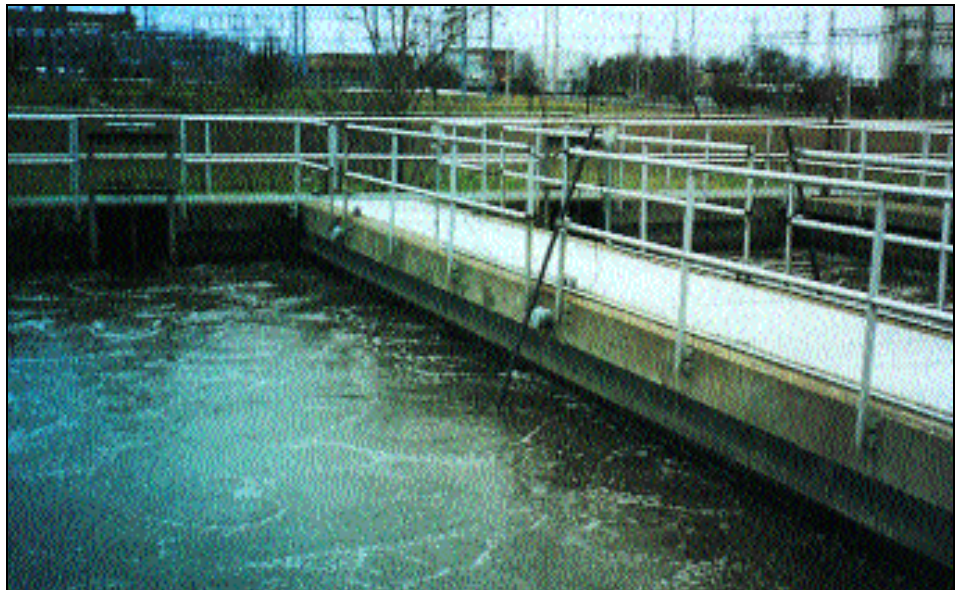
Dissolved oxygen sensors at the Oswego, N.Y. West Plant have an adjustable set point that automatically regulates the flow of air into the diffuser system.
